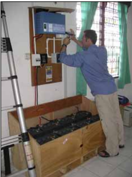
This large system can automatically switch between town and solar power
